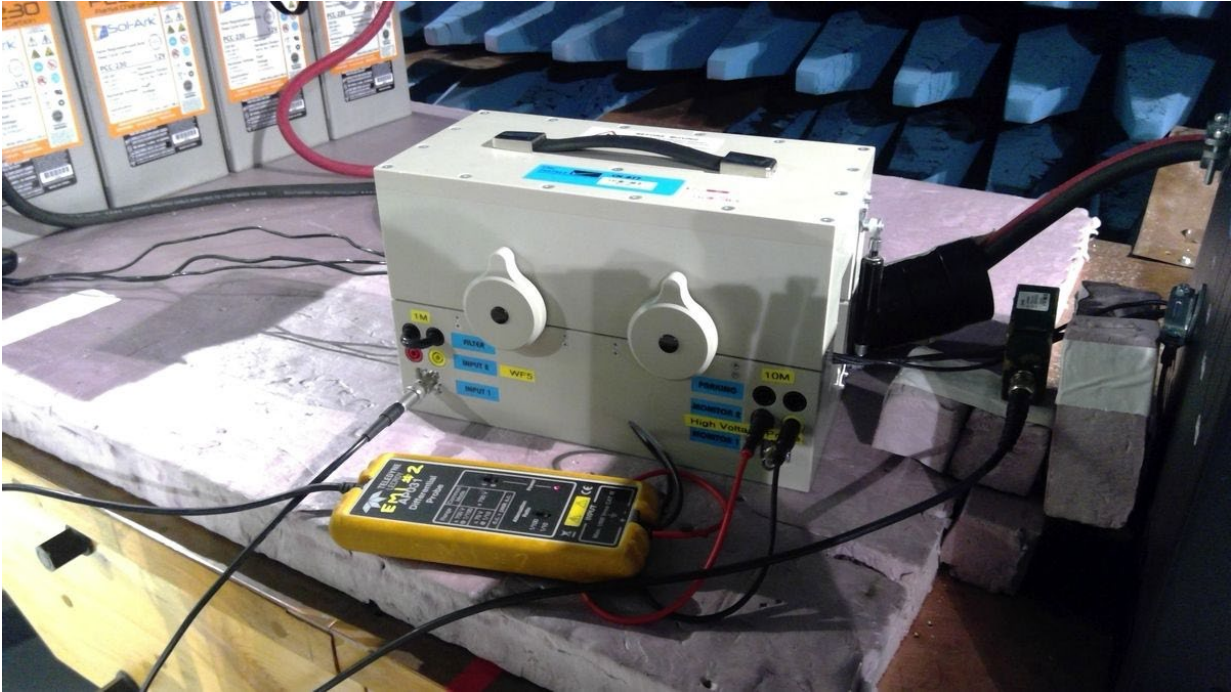
3 CS117 Active AC Bundle Testing
