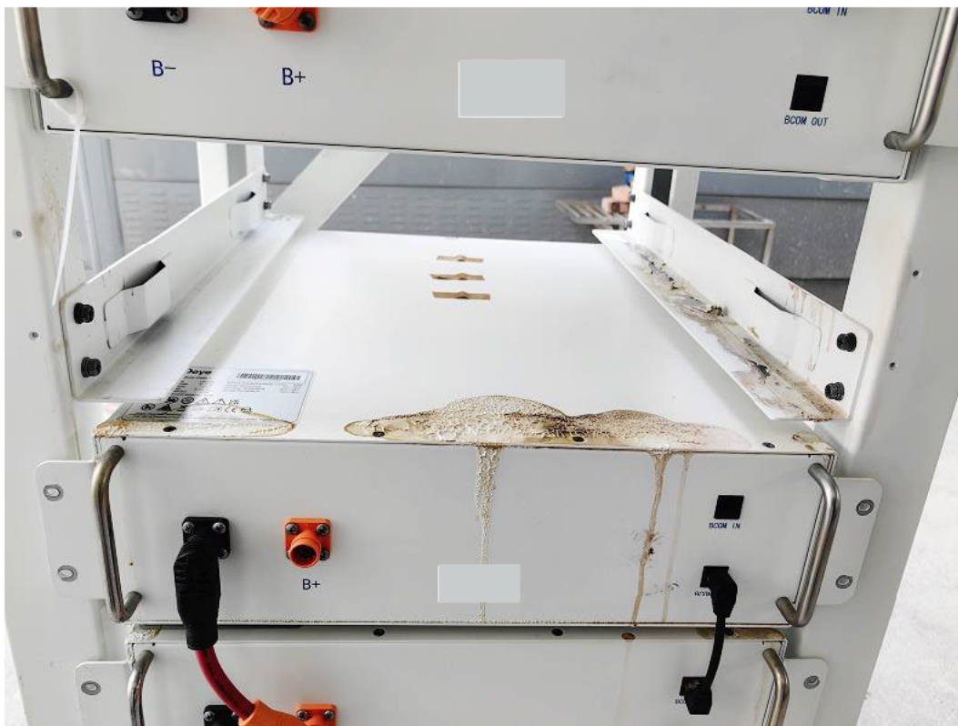
Figure 20. Photo 04 of initiating BESS unit after test.
