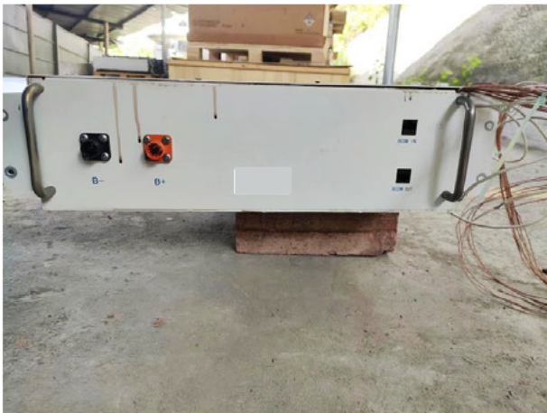
Figure 21a. Photo 01 of initiating battery module after test.
