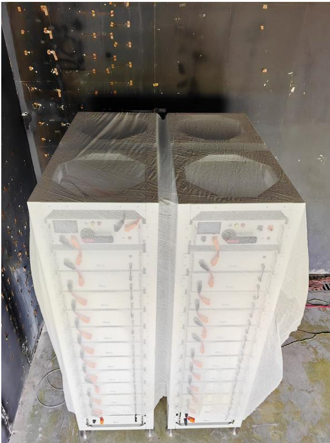
Figure 15. Photo 01 of initiating BESS unit and target BESS units after test.
