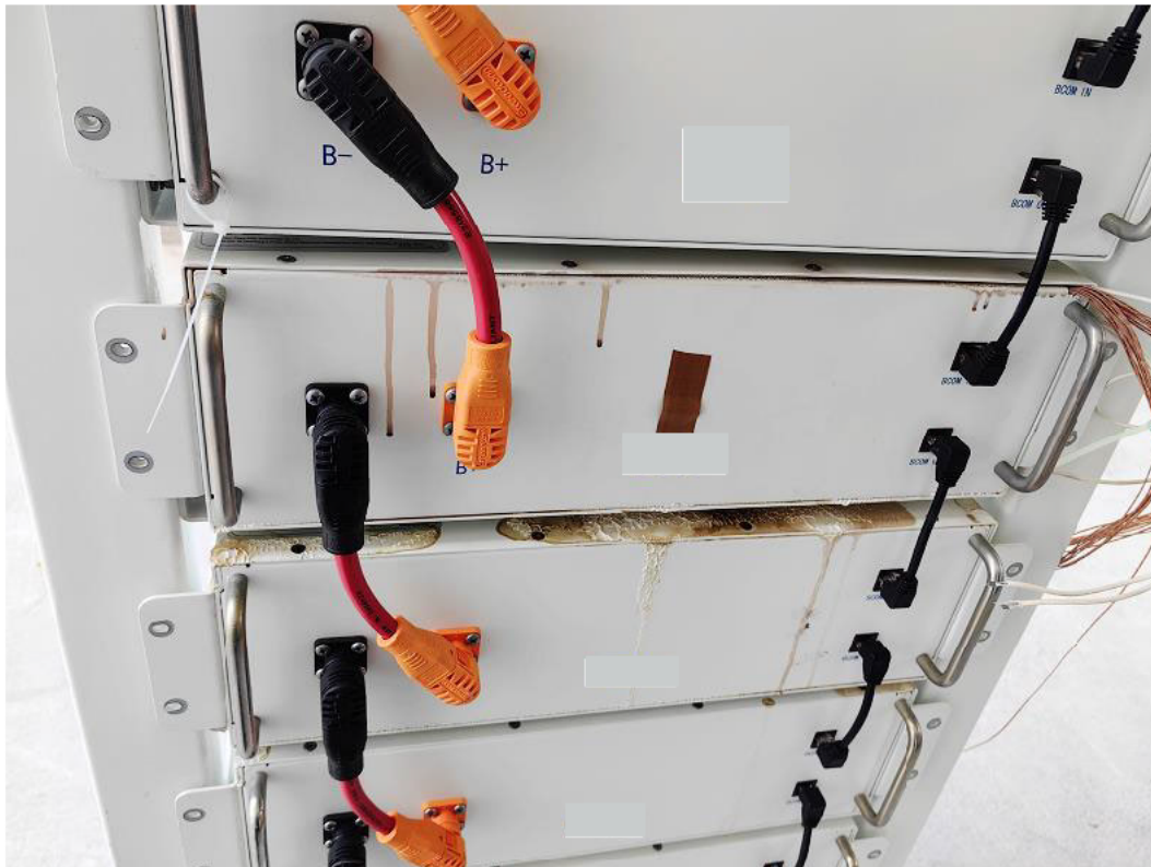
Figure 19. Photo 03 of initiating BESS unit after test
